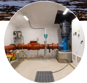
The pump house is the heart of the operation, securing all mechanical and electrical systems.
