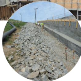
Shotcrete was an ideal choice for stabilizing the hillside, which has a 2:1 slope.
