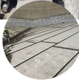
The FLSmith Ful-Floor™ center discharges to the tunnel.
