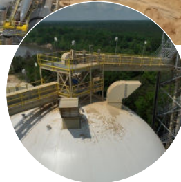
A diverter at the dome apex directs pellets to the desired dome for storage.
