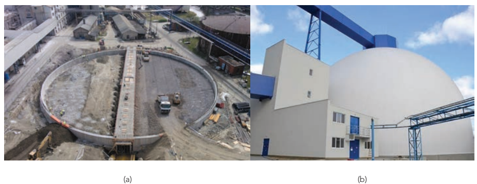
Figure 1: Pictures of the sugar silo: (a) Under construction, and (b) After completion
